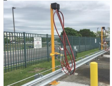
CLEAN & RENEWABLE ENERGY
